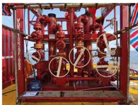
Figure 4—Dual-pot sand filter was mobilized and tied-in at flowline using temporary piping as part of temporary surface assurance package during initial well flowback.
